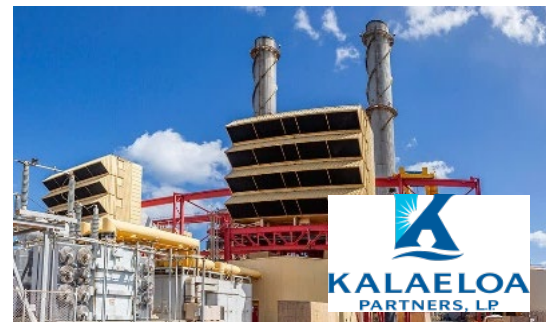
RENEWABLE FUEL COGENERATION
